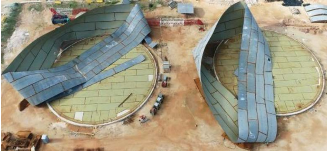
ULSD Tanks destroyed by Typhoon Mawar, May 25, 2023
